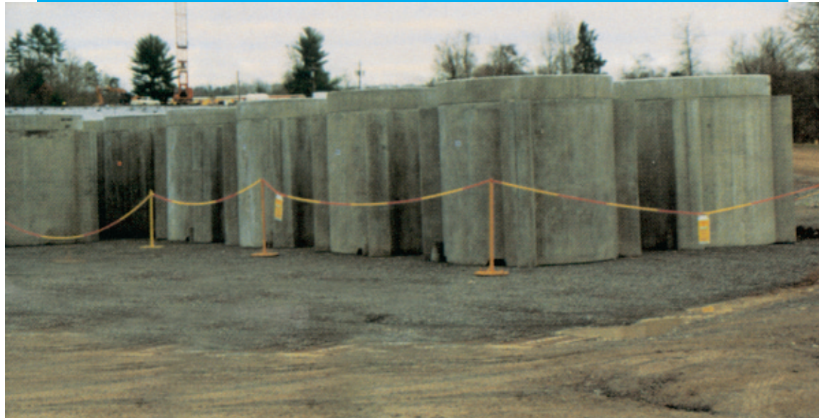
These completed tanks are ready for storing nuclear waste.
